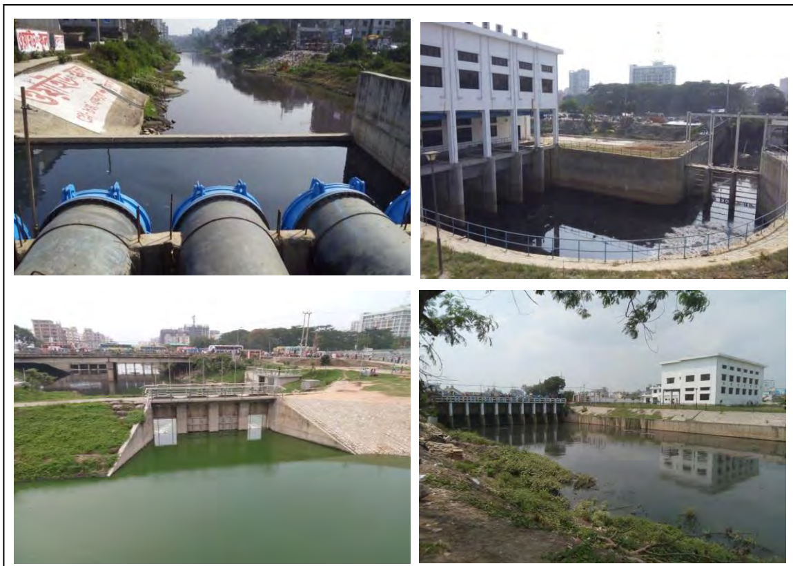
Figure 4.7: Rampura Pump house Area
