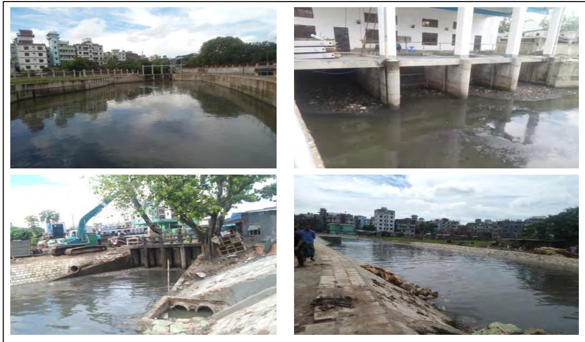
Figure 4.6: Maniknagar Pump house Area
