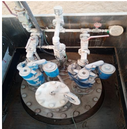
Figure-23: Chemical Delivery pump.
