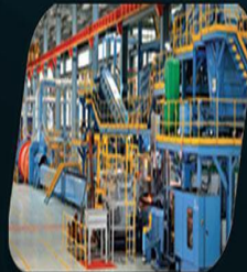
Green Sand Pressure Molding Line
