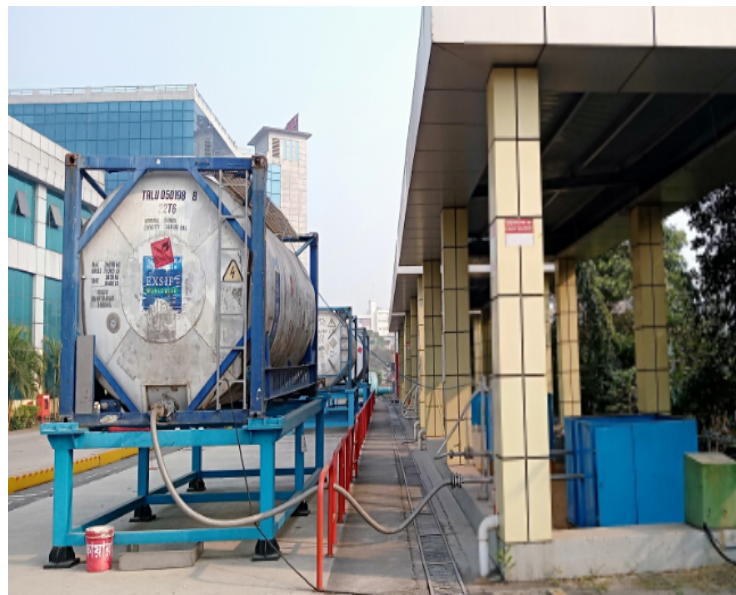
Figure-20: Chemical Loading On The Underground Storage Tank , From the Base of the Container.
