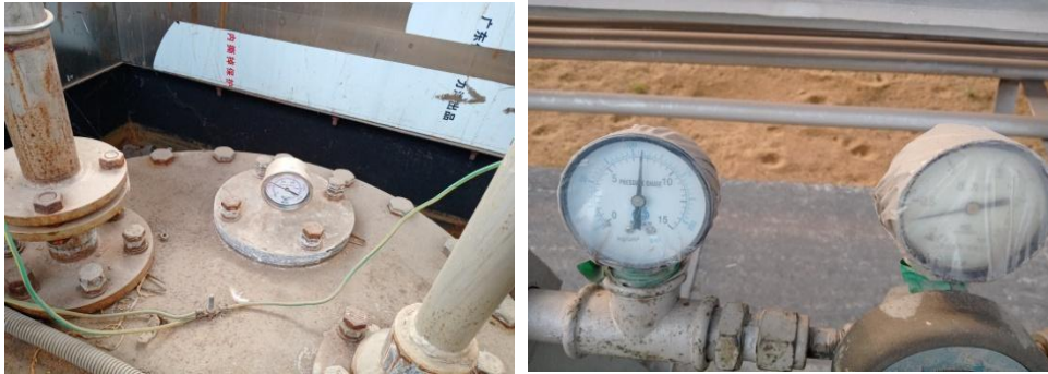
Figure 07; Nitrogen Pressure Gauge Meter.
