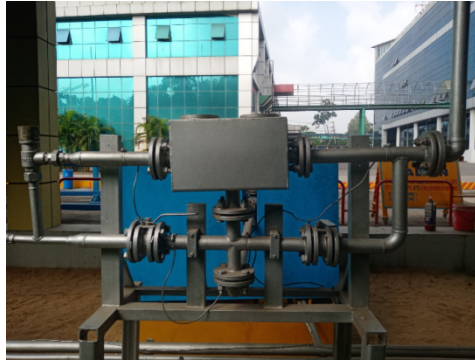
Figure 09; Safety Weight Valve.
