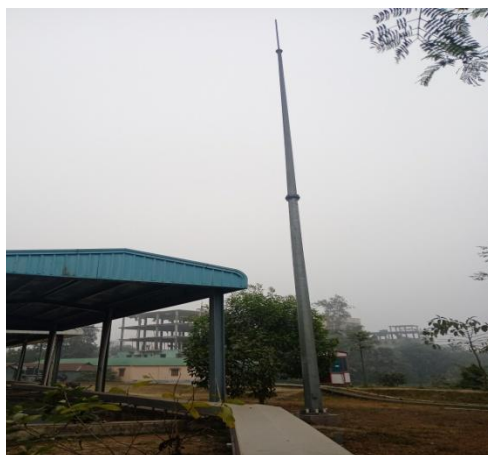
Figure:04; Lightning Arrester.
