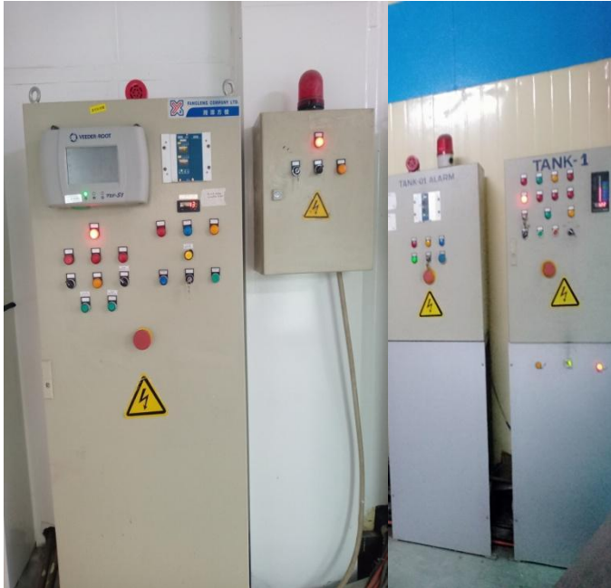
Figure-22: Font View Of The All Control Panel.
