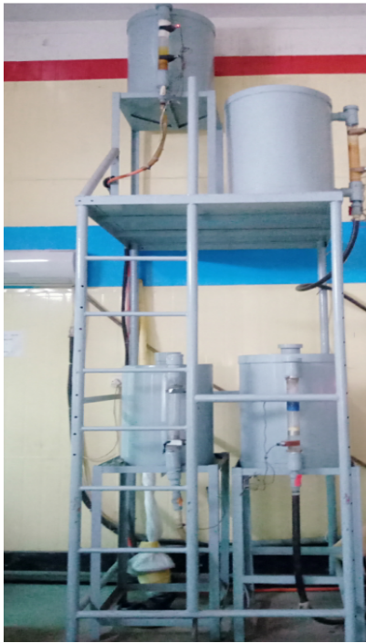
Figure : 05; The Glycol Storage Tanks.
