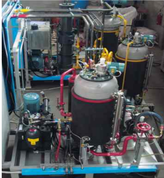
Figure-20: Picture of The C-5 Chemical Mixing Tank.
