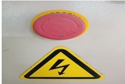
Figure 15; Emergency Push Button Switch.
