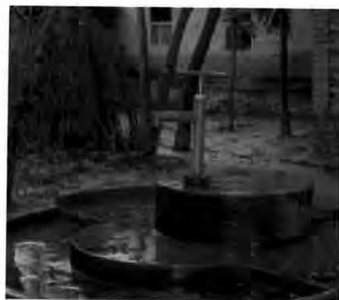
Fig. 2.10: Dug well with Tara pump
