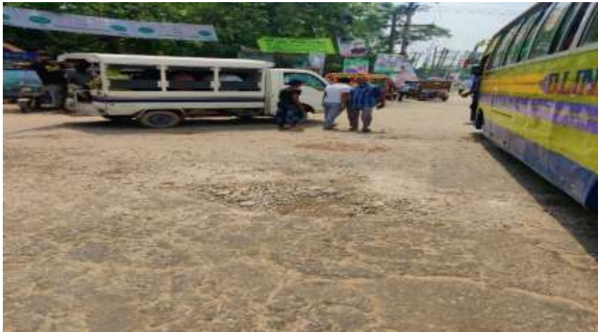
Figure 4.8.1: Poor Road Surface
