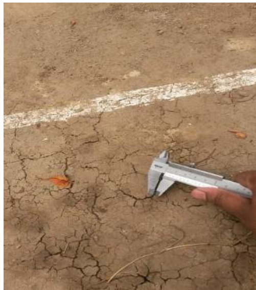
Figure 3.50: Measuring the crack width
