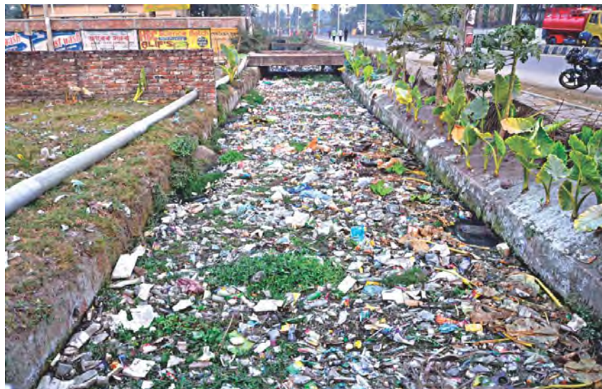
Figure 6.14 Waste Disposal on Drain
