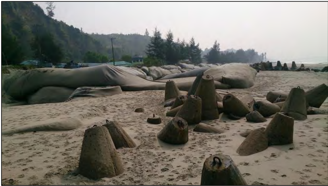
Figure 4.5: Damaged protection system at Himchari point, Cox-Bazar
