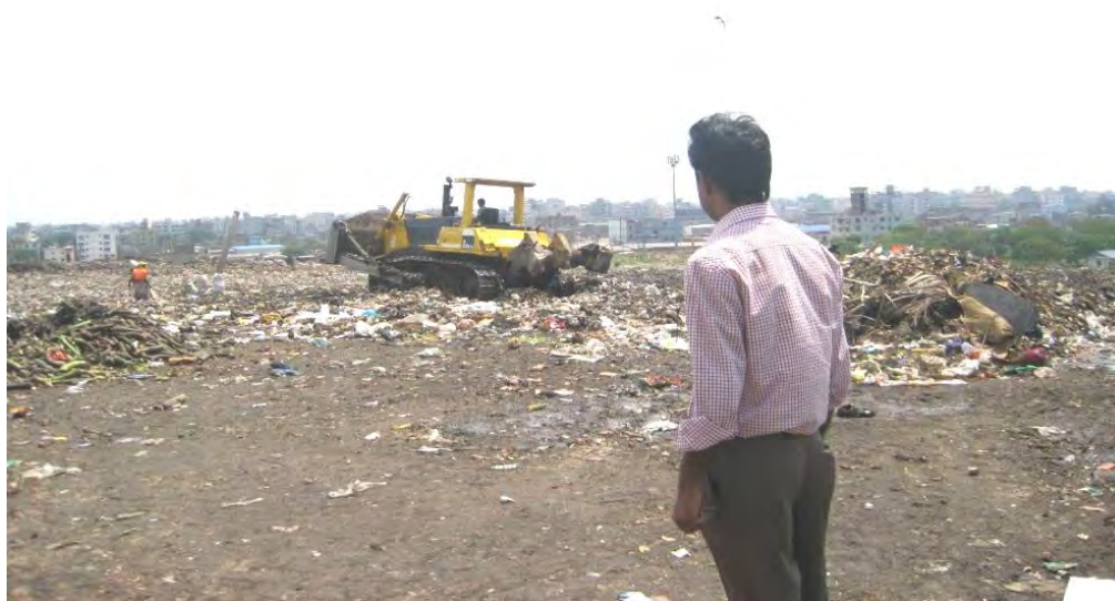
Photograph-A6: Spreading of Waste using Pay Loader was found during Field Survey in April 2013 at Matuail Dumping Site under DSCC
