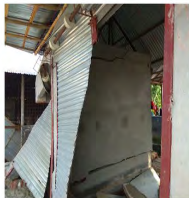
6. n) Erosion affected business shop
