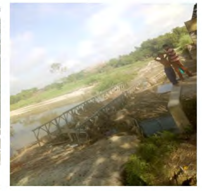
6. l) Collapsed bridge
