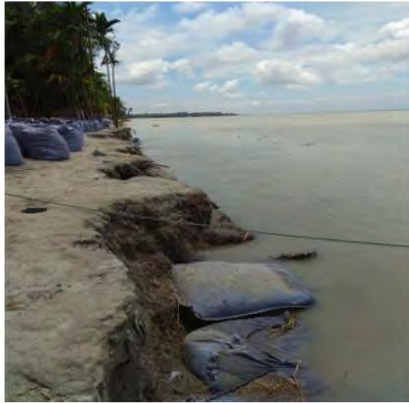
2. a) Bank erosion
