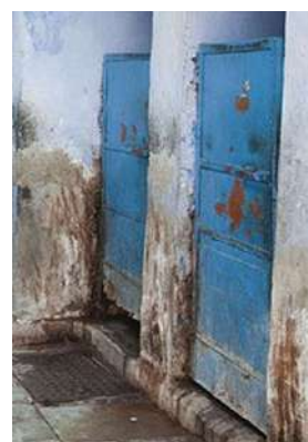
Figure 4.9: Poor Situation of the Female Separate Toilets in Milk Vita Khalpar Basti
