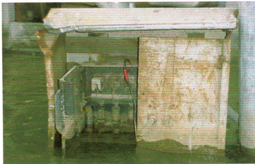
Photograph 6.5 Showing the waterlogged power grid
