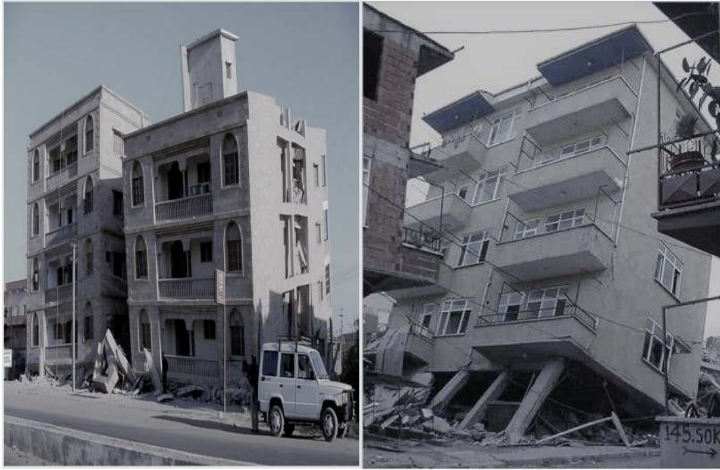
Figure 2.6: Formation of soft storey, Bhuj earthquake, India, 2001
