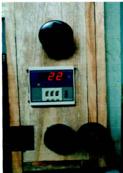
Fig. 3.11: Switch board of the dryer
