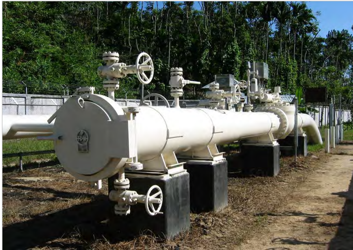
Fig.B.3: A Pig Receiver of NS 24" Pipeline
