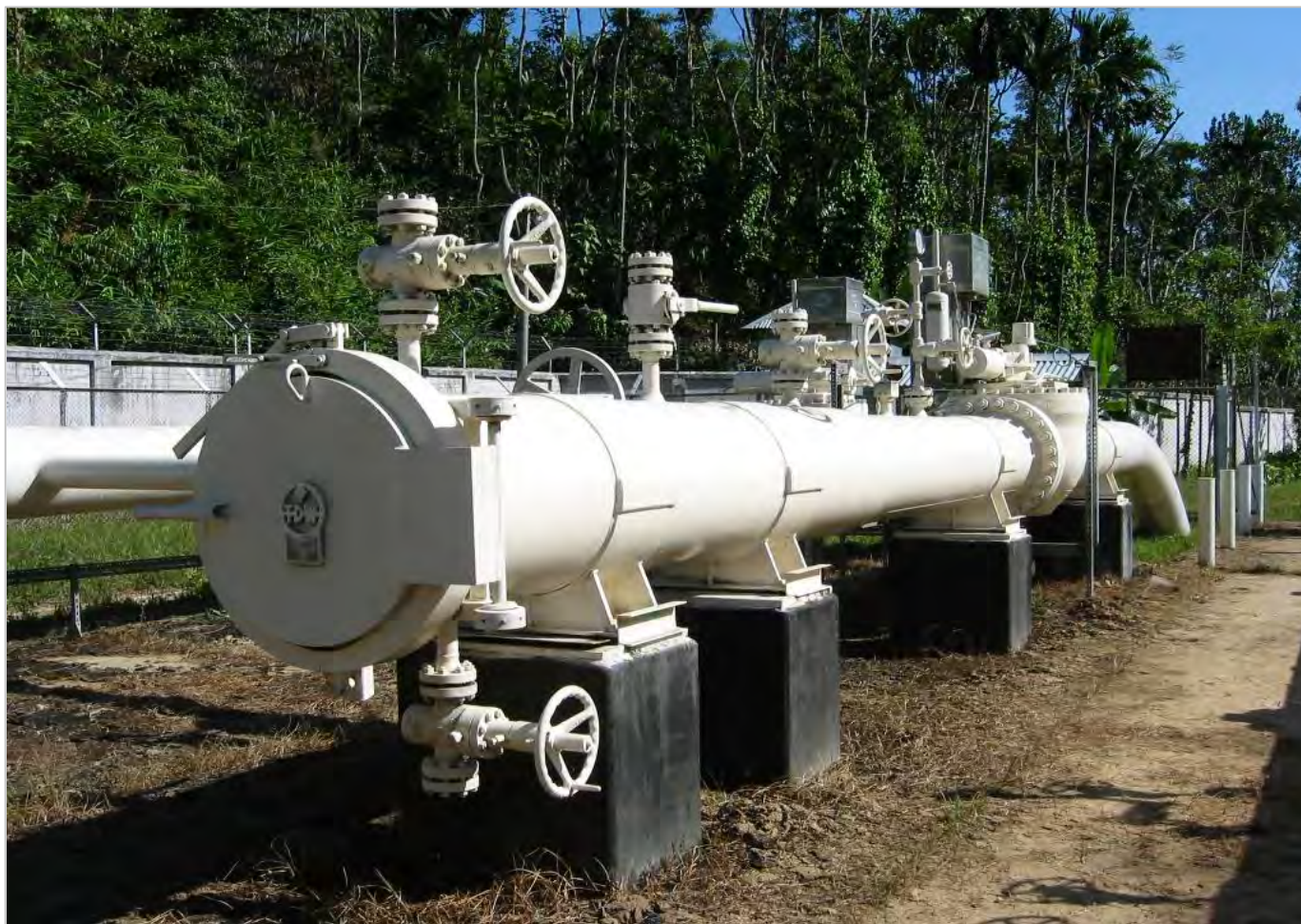
Fig.B3: A Pig launcher of Ashuganj-Bakhrabad 30" Pipeline
