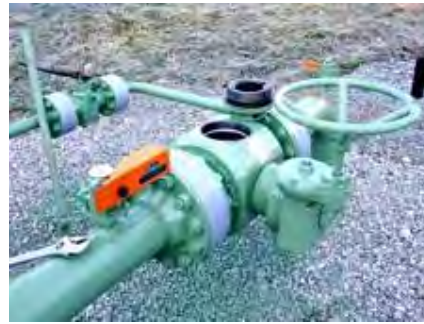
4" Pig Receiving Valve with gear operator and Hi-T Pigalert pig detector.
