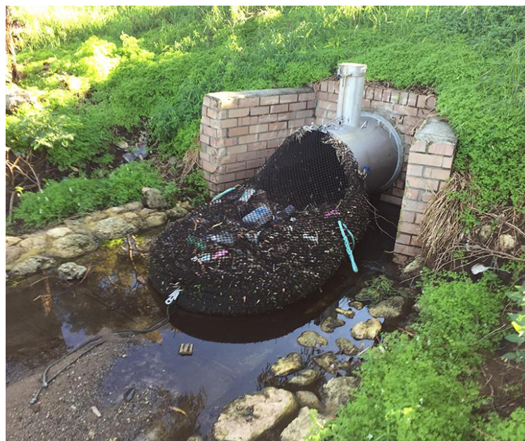
Figure 31 Safe our environment and rivers from drain waste by using net
