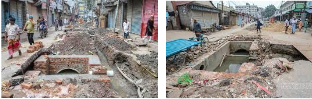
Figure 28 Subsurface drain in Naya Bazaar, Dhaka
