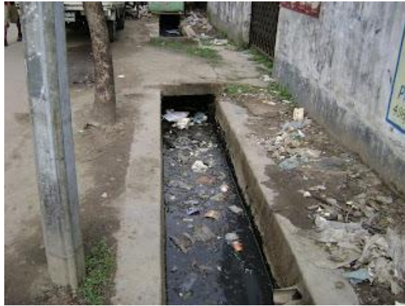
Figure 26 Ashulia Bazaar side drain
