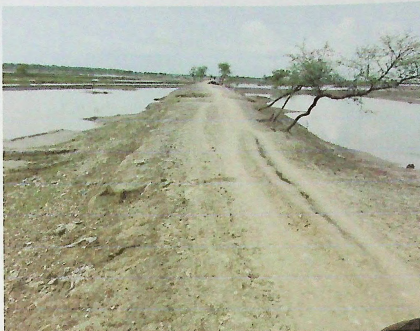
Inaccessible road, Ashashuni, Satkhira, Bangladesh
