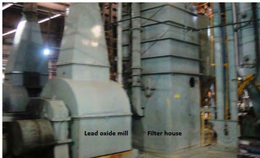
Fig. 4.2: Main functional machines for lead oxide production system
