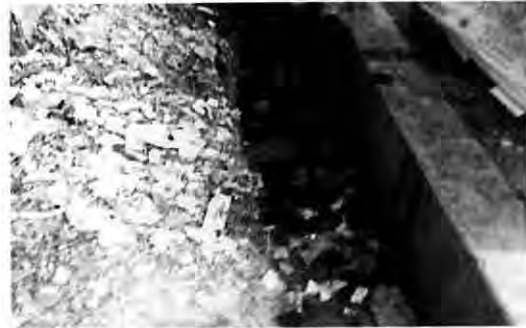
Plate 4.10 HCW clogs sewers of Khulna General Hospital
