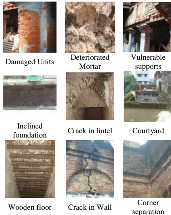
Fig. 5: Defects and extent of damages in Shakhari Bazar.
