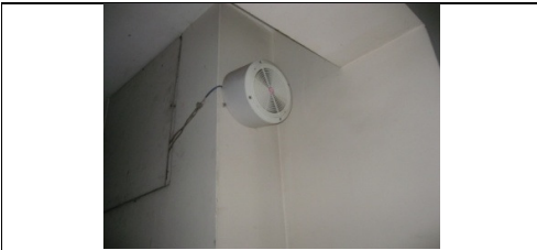
Fig 4.8: Fire alarm in an apartment of Nasirabad residential area.
