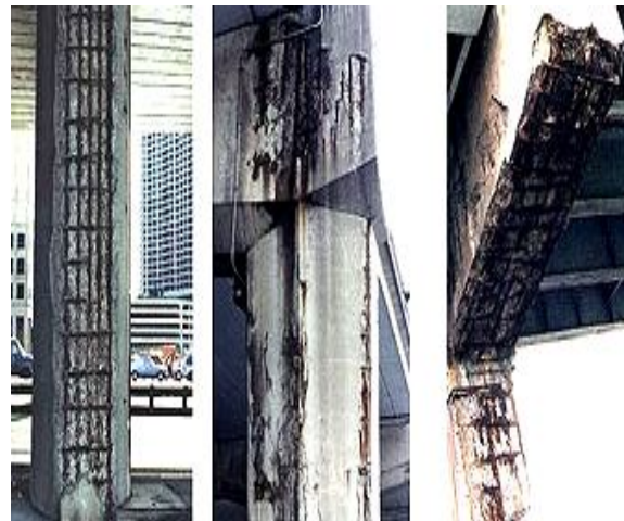
Fig. 11: Rusted and exposed concrete reinforcing steel bars because of severe corrosion.
