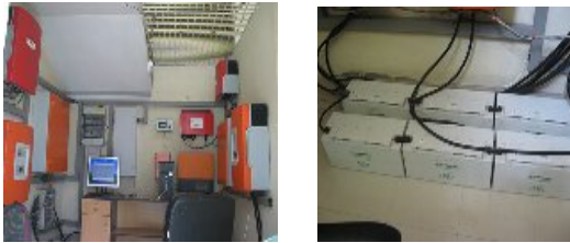
Fig. 2: Control room and batteries.
