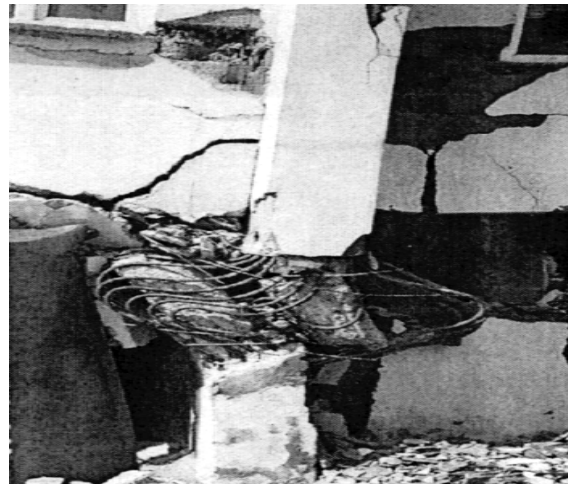
Fig: 10. Column failure due to insufficient proportion of low strength highly ductile reinforcing steel bars.
