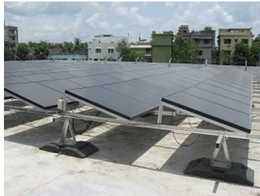
Fig. 1: PV panels installed on the roof
