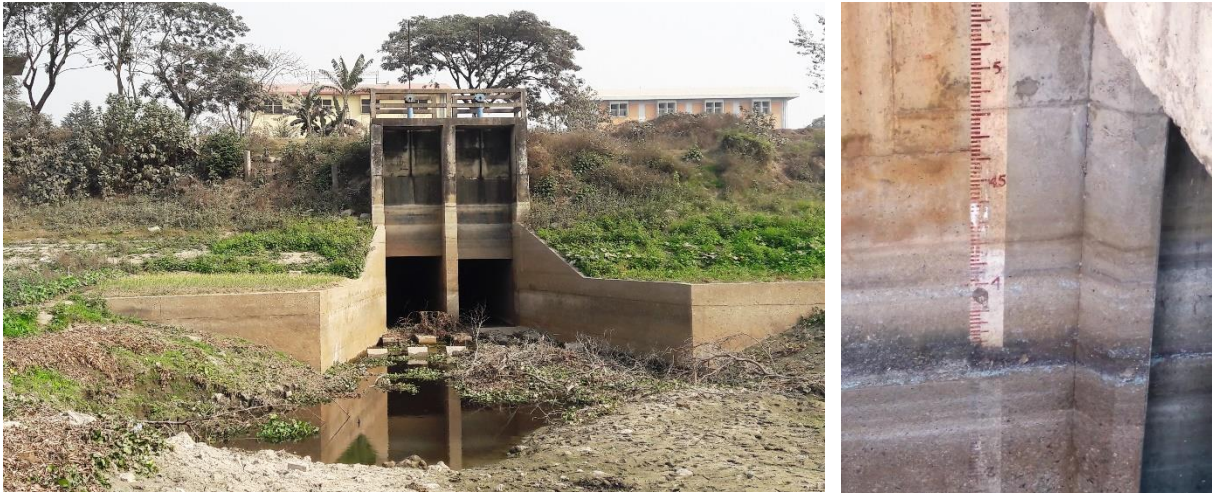
Figure 5-17: Goranchatbari Pump Station (River Side) & pump start level.
