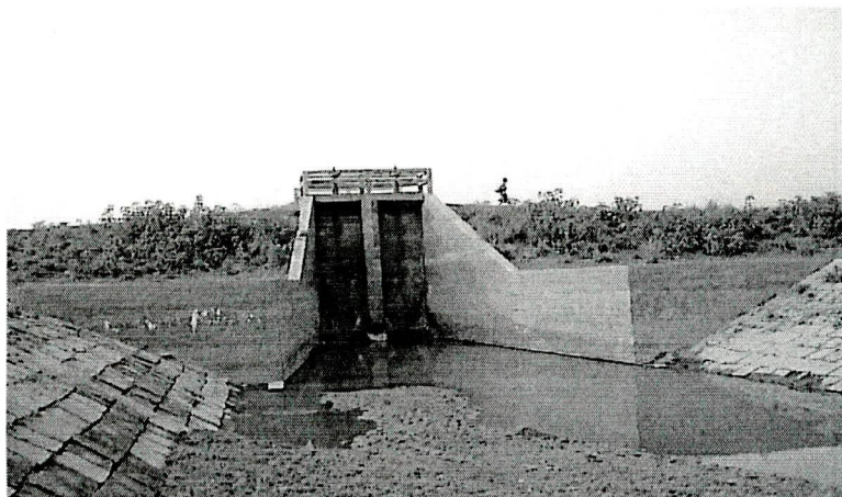
2 Vent Regulator, Dulia Satbila Sub Project
