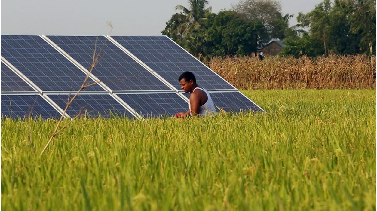
Figure 1.3: Solar Panel situated the paddy field
