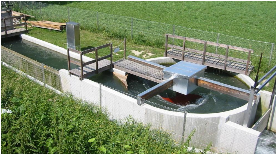
Figure 2.14: Micro/Mini Hydro power plant
