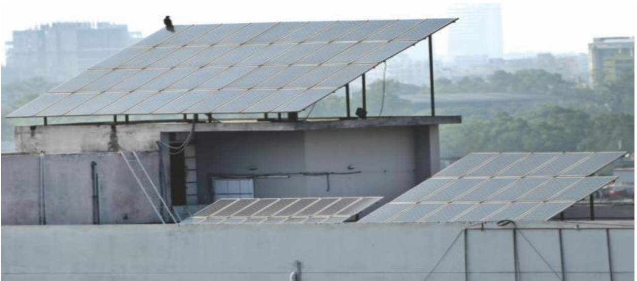
Figure 2.2: The SHS system in town area
