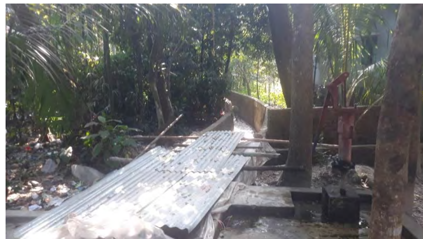
Image C44: Uncovered RCC drain near Sultan fokir mazer (south), Bauphal municipality
