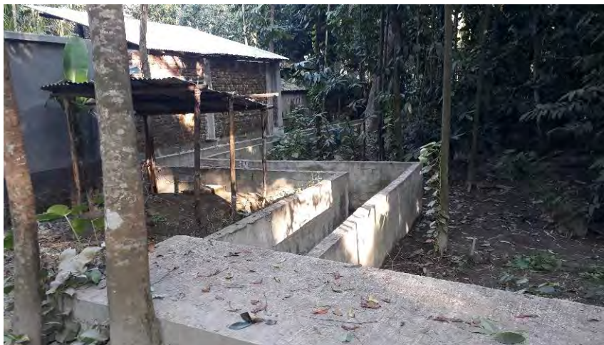
Image C53: Uncovered RCC drain near Md Waydul mia bari, Bauphal municipality
