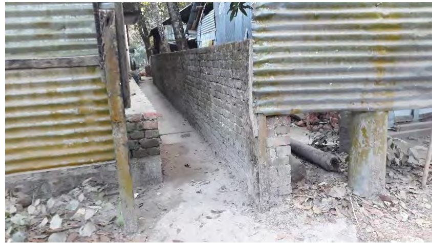
Image C60: Hole in covered RCC drain near Monir master bari, Bauphal municipality
