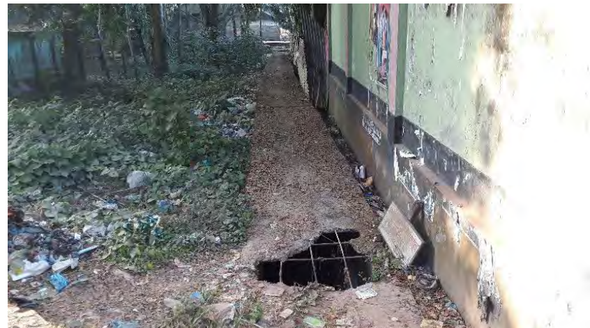
Image C56: Hole in covered RCC drain near Daruet sunat, Bauphal municipality
