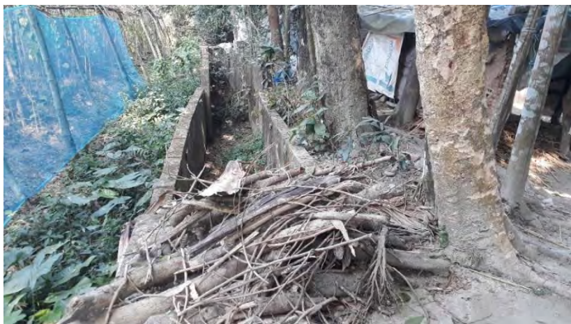
Image C41: Uncovered RCC drain near Nitaipalli bari, Bauphal municipality
