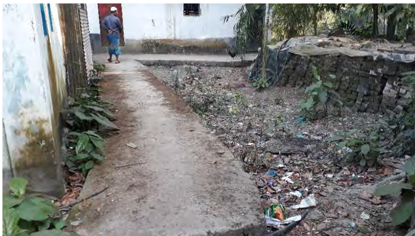
Image C57: Hole in covered RCC drain near Daruet sunat, Bauphal municipality
