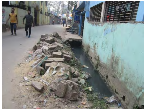
Image C22: Poor drainage system at Pathanbari road in Feni municipality
