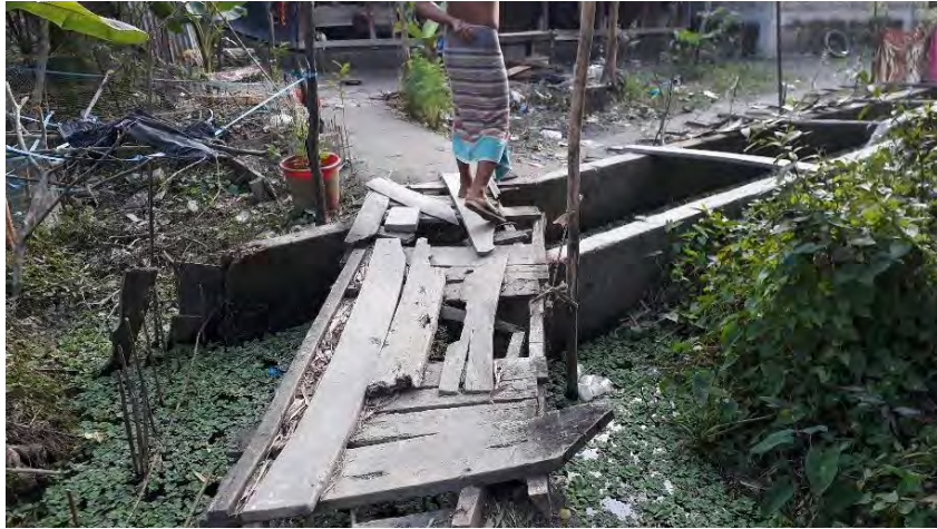
Image C59: Uncovered RCC drain near Sarderbari to Sadhu Howlader bari, Bauphal municipality
