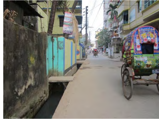
Image C21: Uncovered drain at Pathanbari road in Feni municipality
