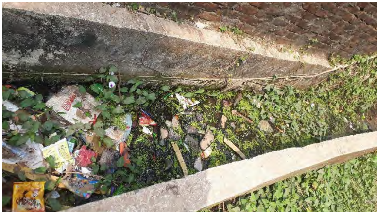
Image C29: Solid waste dumping at RCC drain near Biraj Majumder Bari in Feni municipality
