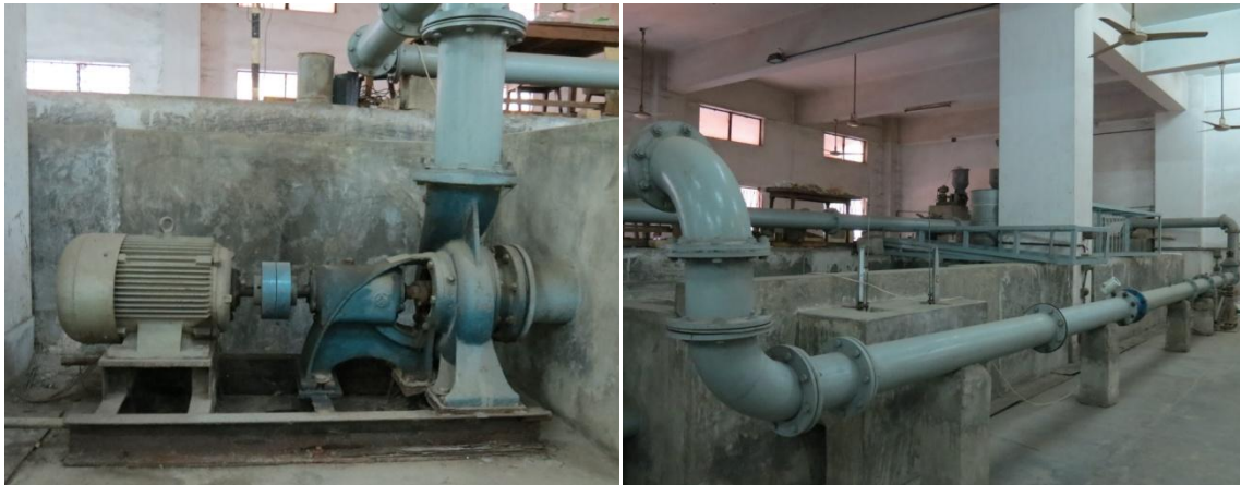
Figure 4.7: Pump and pipe line
