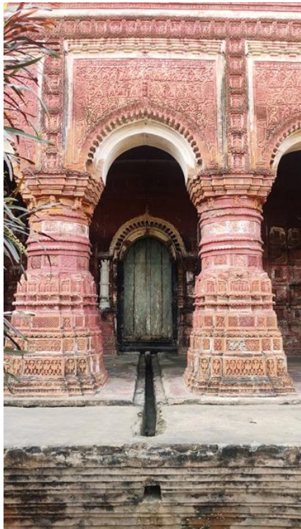
(c) Drainage System from main Sanctum
